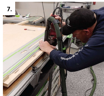
7. Use the center marks for the Tenso connectors and make plunge cuts
