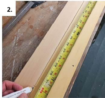
Lay out and match connector slots on edge of jamb leg and back side of casing
